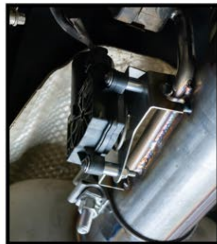
VALVE INSTALLED SHOWN ABOVE
